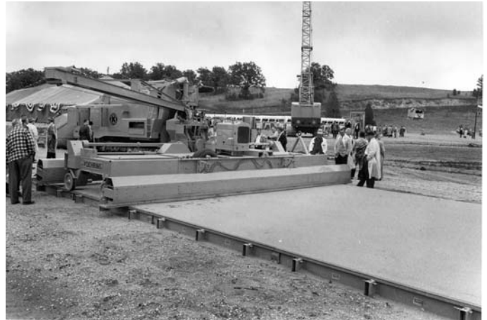
Paving forms provided by MFC were part of a demonstration of the world's largest mobile-paver - the "Tribatch" - at a 1961 exhibit on the Koehring Company test grounds.
