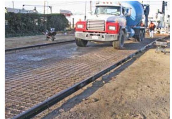
The city used six-inch steel forms from Metal Forms Corporation. Reinforcing wire mesh shown here was pulled up into concrete once poured.
