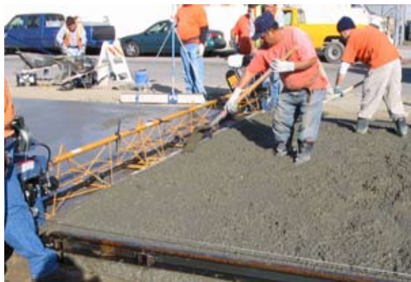
Workers ahead of screed controlled concrete level with shovels and pulled wire mesh, visible at right, up into center of slab thickness for maximum reinforcement.
